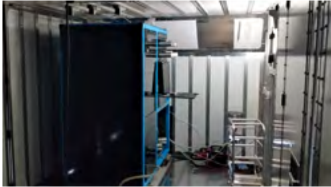
Integration of the upgraded OSI SAUNA system into the new flight pod.
