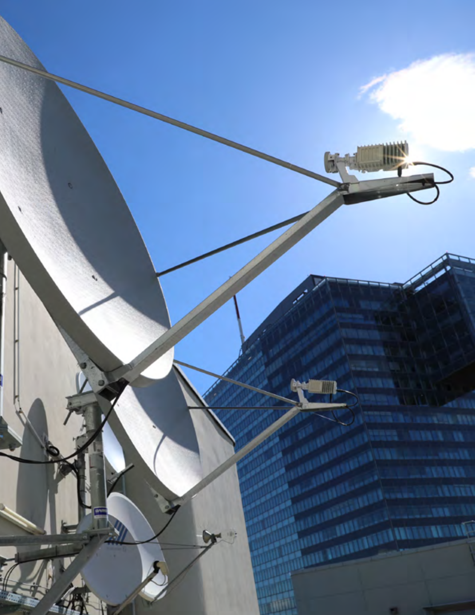
GCI III installation on the roof of the Vienna International Centre, Austria.
