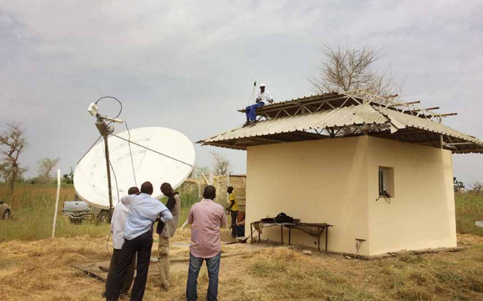
A team of technicians working to fix the VSAT antenna. In the background an operator is installing the GPS receiver.
