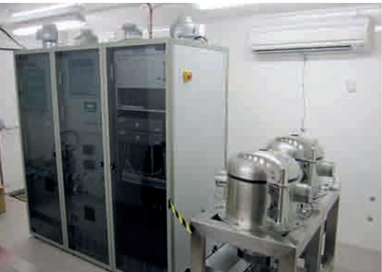
The SAUNA noble gas measuring system at radionuclide station RN68, Tristan da Cunha (United Kingdom).
