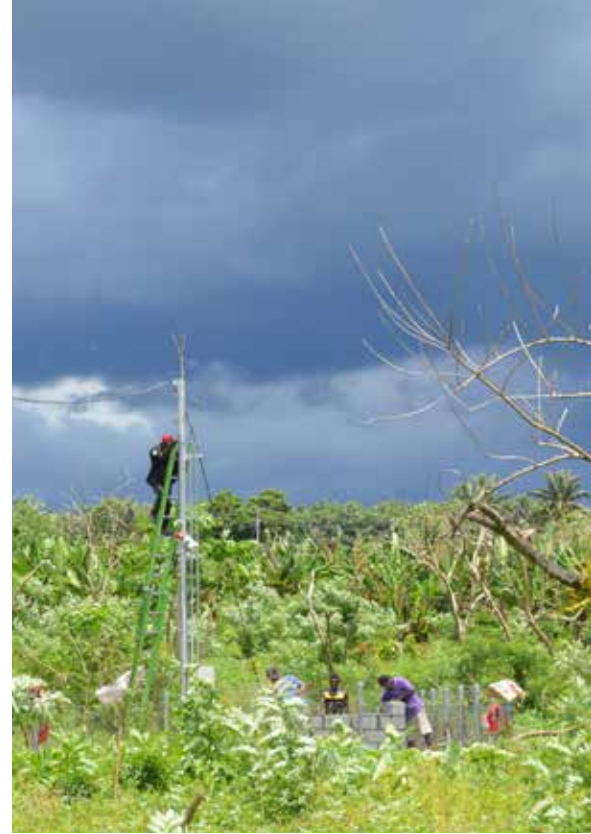
RVO workers relocating fibre optic cables to enable the eventual transmission of data all the way back to Austria.
