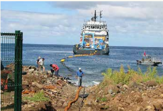
HYDROACOUSTIC STATION HA03, JUAN FERNANDEZ ISLAND, CHILE, SEEN HERE DURING CONSTRUCTION. THE STATION WAS DESTROYED BY A TSUNAMI IN FEBRUARY 2010 THAT DEVASTATED THE ENTIRE ISLAND.
