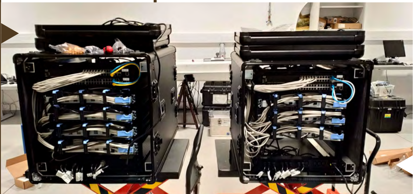
► Rear view of new working area and receiving area servers.
