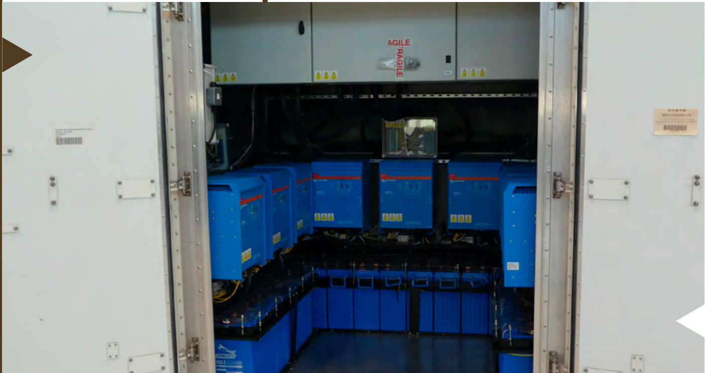
► View of the hybrid power unit, integrated in an OSI rapid deployment pod to support field power distribution with solar energy at the base of operations.
