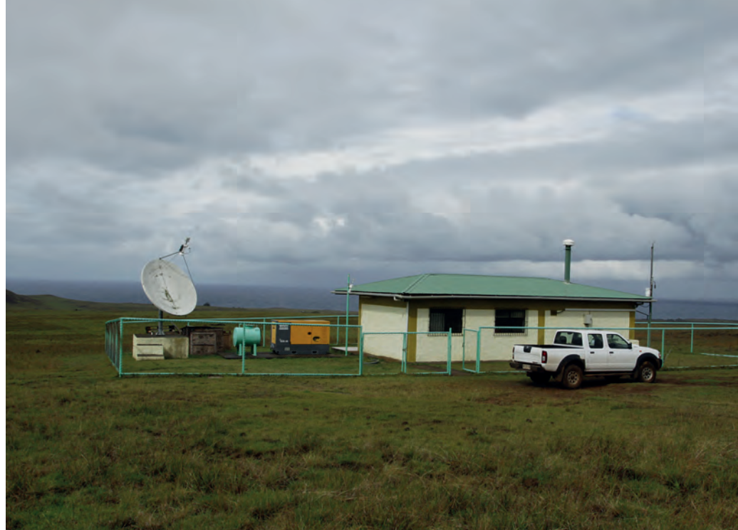
Upgrading radionuclide station RN19, Hanga Roa, Easter Island (Chile)
