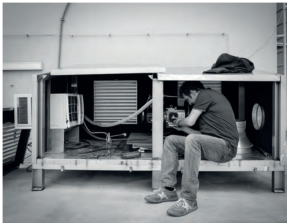
Repair of a noble gas system compressor at the Vienna International Centre
