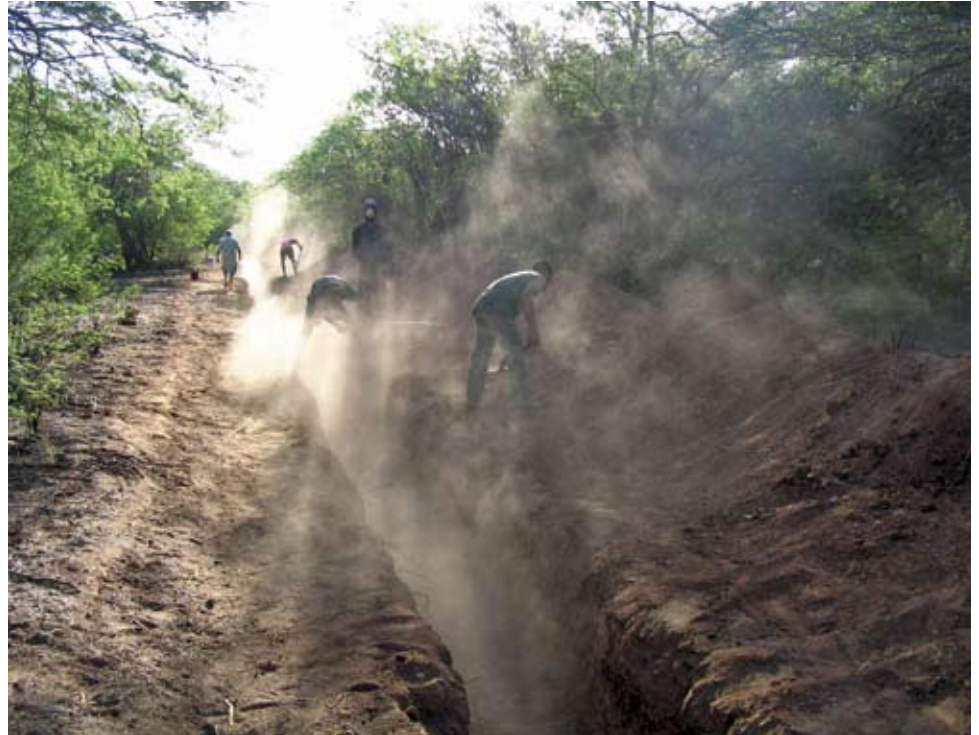
DIGGING THE TRENCHES FOR THE INFRASOUND ELEMENTS OF IS11, CAPE VERDE, DECEMBER 2006
