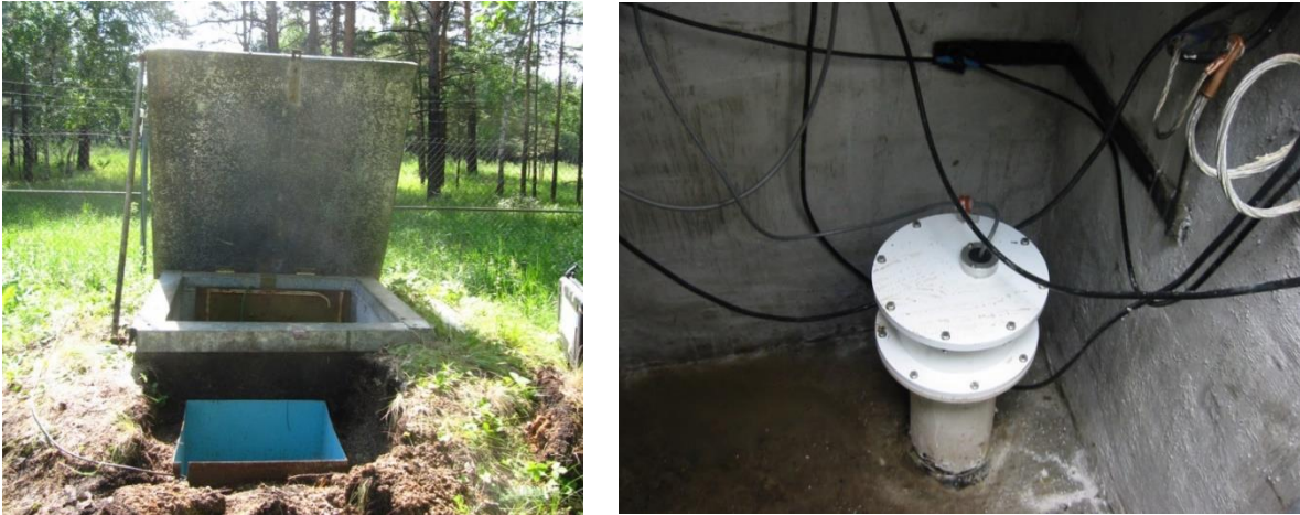
Figure 2. External view of an existing vault (left) and borehole termination inside an equipment vault (right).
