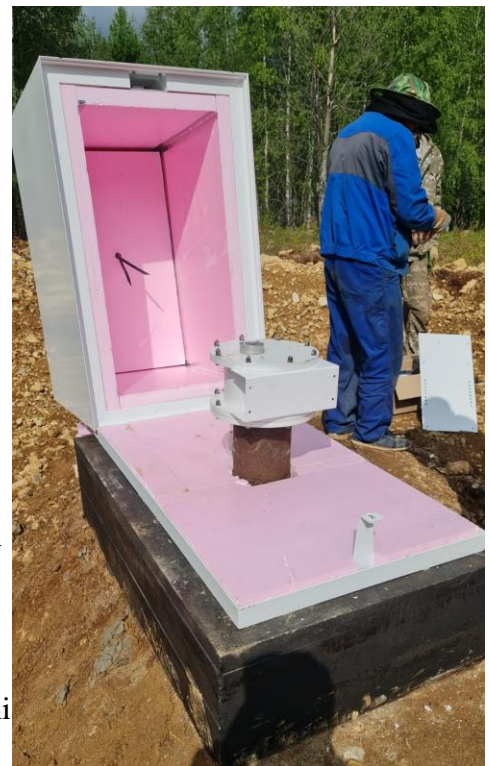
Figure 4. Example of a borehole enclosure, closed and
