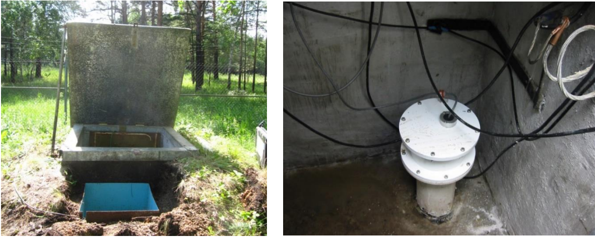
Figure 2. External view of an existing vault (left) and borehole termination inside an equipment vault (right).
