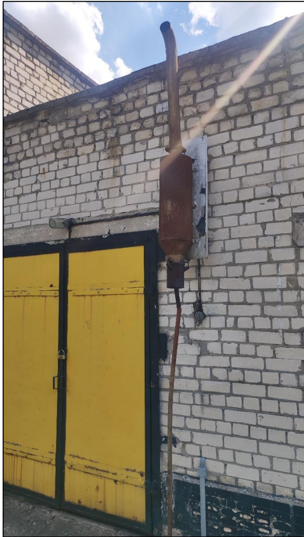
Left Photo: Exhaust piping #1 outside of the Generator Building
