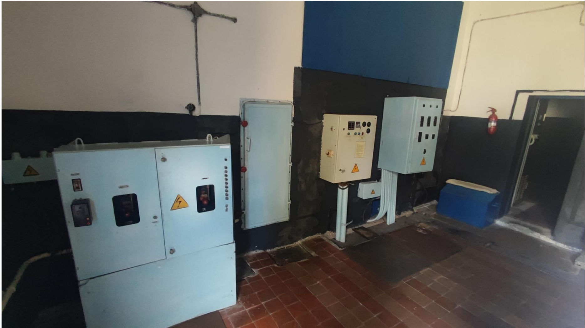
General Layout of Generator Building Electronic Boxes
