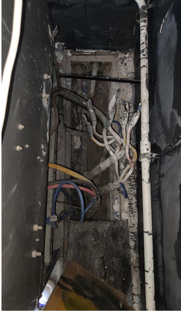
Degraded Electrical Wiring beneath DG-2
