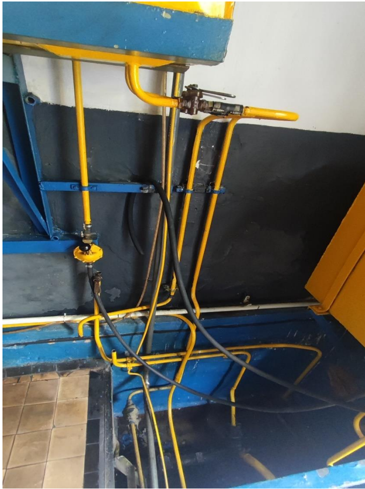
Left Photo: Manual Fuel System inside Generator Building Right Photo: Fuel System inside Generator Building (alternate view)
