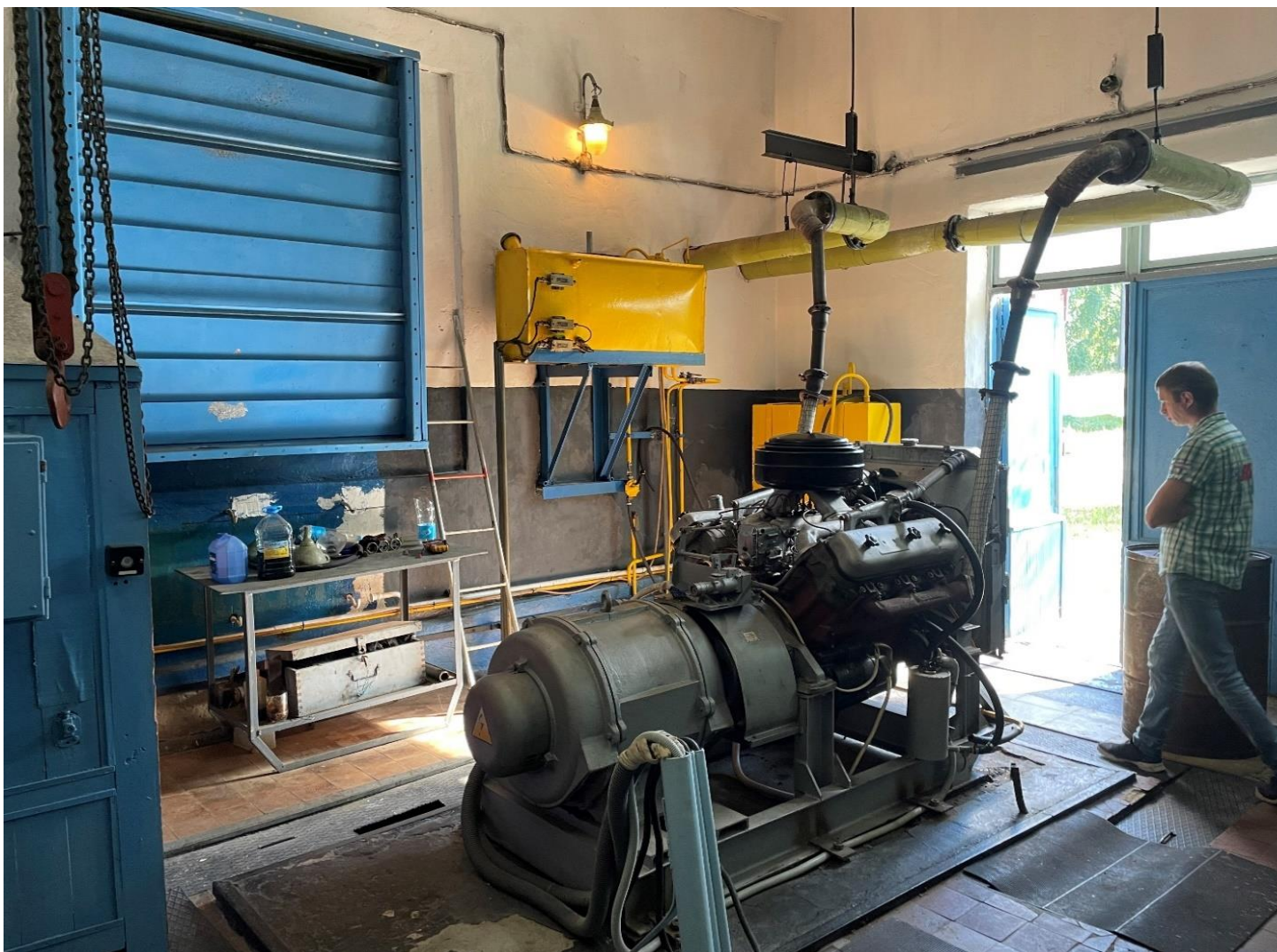
Diesel Generator AD-60/T400 (DG-2 60 kW)
