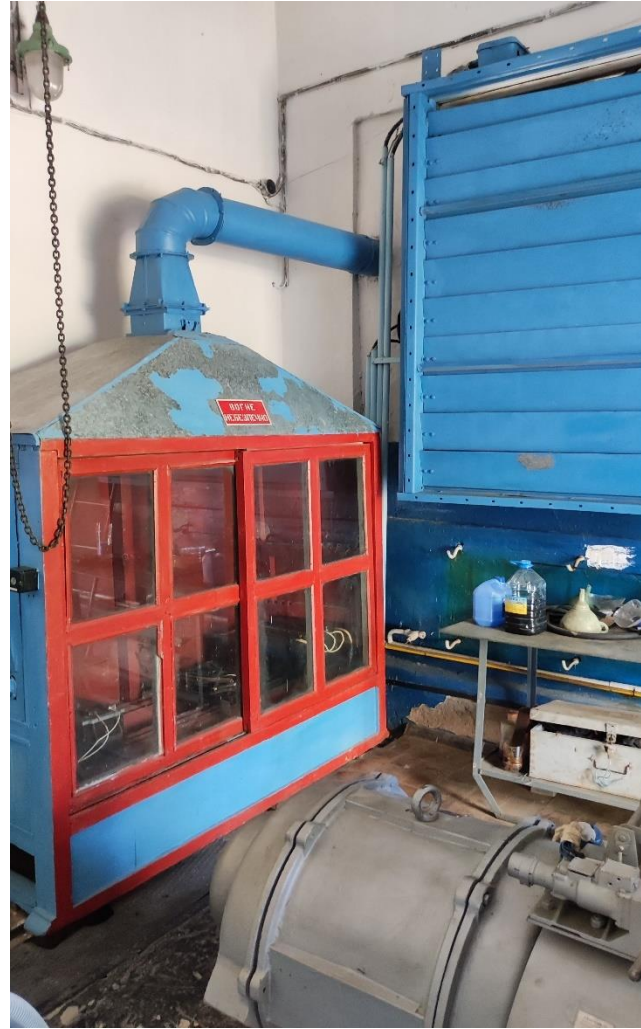
Battery cabinet AD-60/T400.
