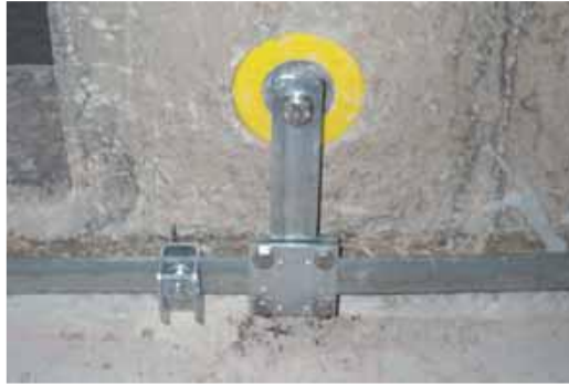
Figure 18: Connection of the ring equipotential bonding bar with the equipotential bonding network via fixed earthing point
