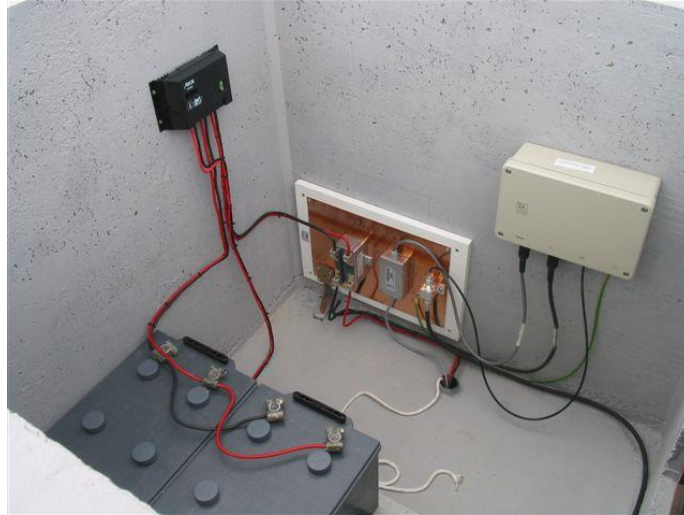
Figure 51: Example of SPDs installed at the entrance of incoming cables to the equipment vault
