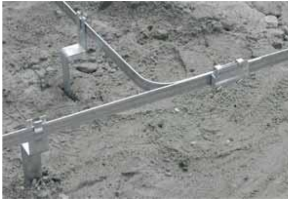
Figure 42: Preparation of foundation earth electrode (spaces ensure that electrodes are enclosed on all sides by concrete)
