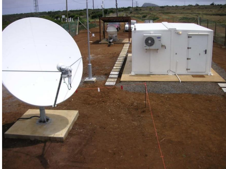
Figure 54: Lightning protection of a radionuclide monitoring station by a metallic tower providing protected volume for the satellite antenna and equipment container
