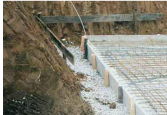
Figure 43: Foundation earth electrode in use
