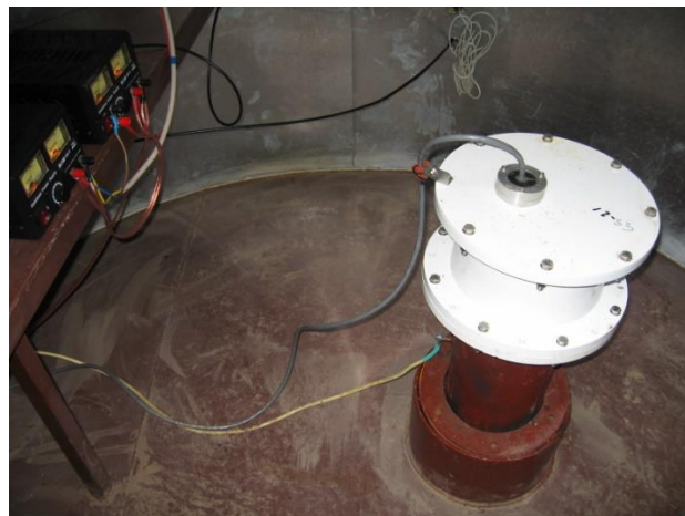
Figure 52: Borehole at an IMS seismic monitoring station with earthing conductor
