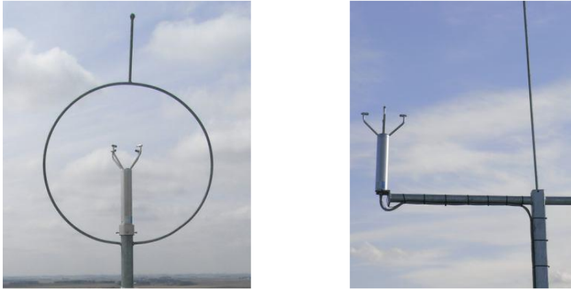
Figure 55: Examples of lightning rods providing sufficient area of protection for a met sensor
