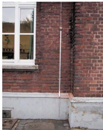
Figure 8: Example of down-conductor mounted on a brick wall
