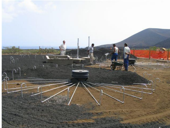
Figure 53: Pipe array at an infrasound station, partly filled by soil
