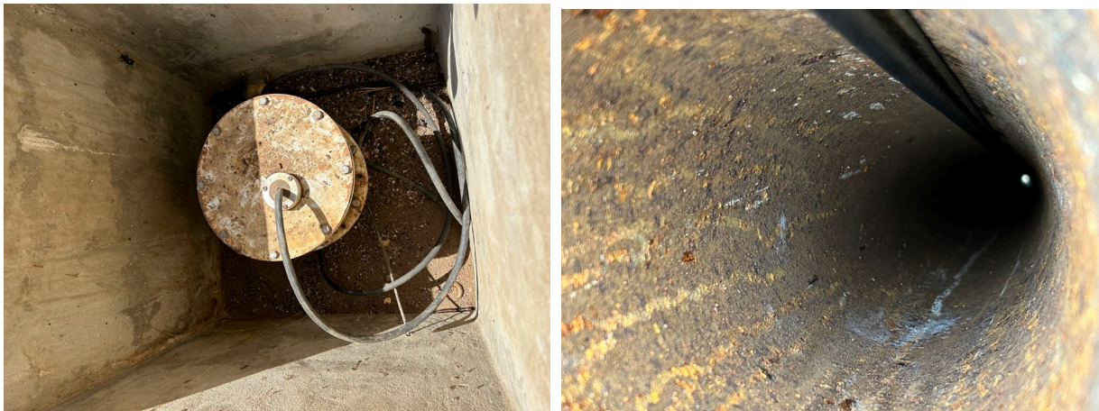
Fig 8.2 Wellhead inside enclosure (left) and inside the casing from top (right)
