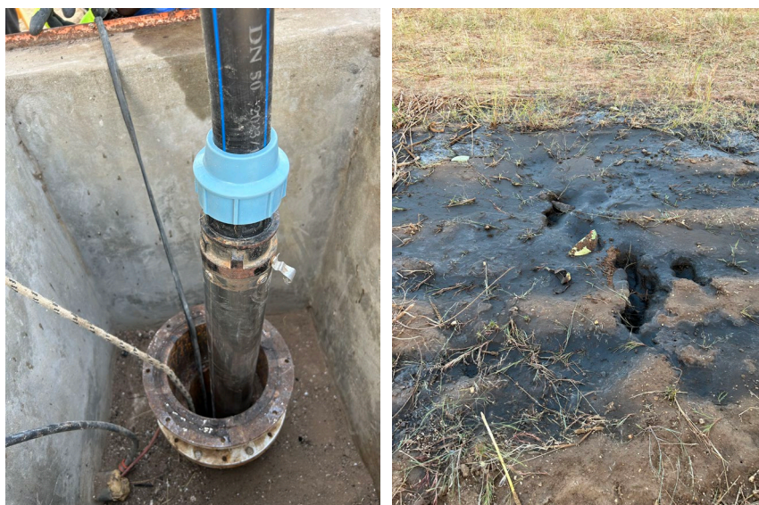
Fig 8.3 Water pumping during cleaning (left) and mud retrieved from the borehole during cleaning.
