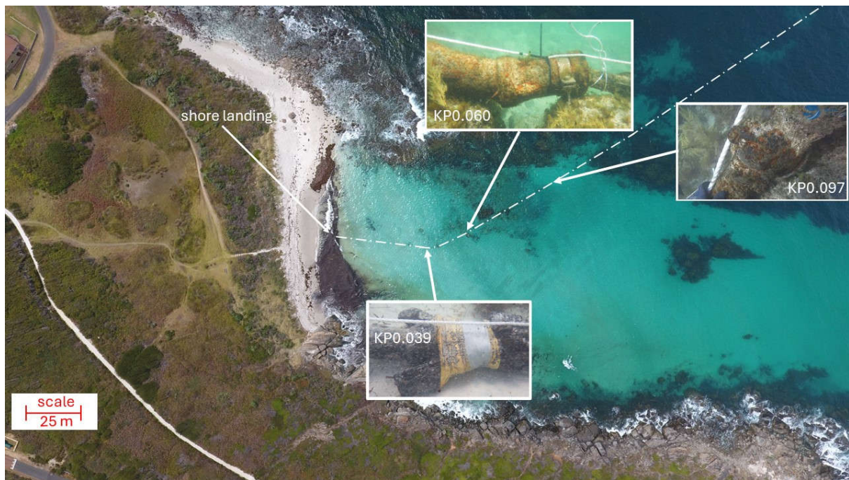
Figure 1: Approximate nearshore cable route (white dashed line); inserts show some of the identified anomalies: sections of failing split pipe at KP0.039 and KP0.060 previously repaired, and newly identified failed split pipe at KP0.097 exposed on a rock, as-found during a December 2023 diver inspection. The status of cable burial seen in the aerial photograph is not the same as status of burial when the three insets were photographed. Note: the background photograph is not oriented northward.
